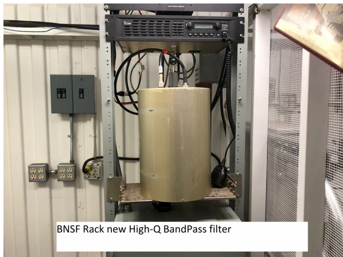
BNSF filter installed
